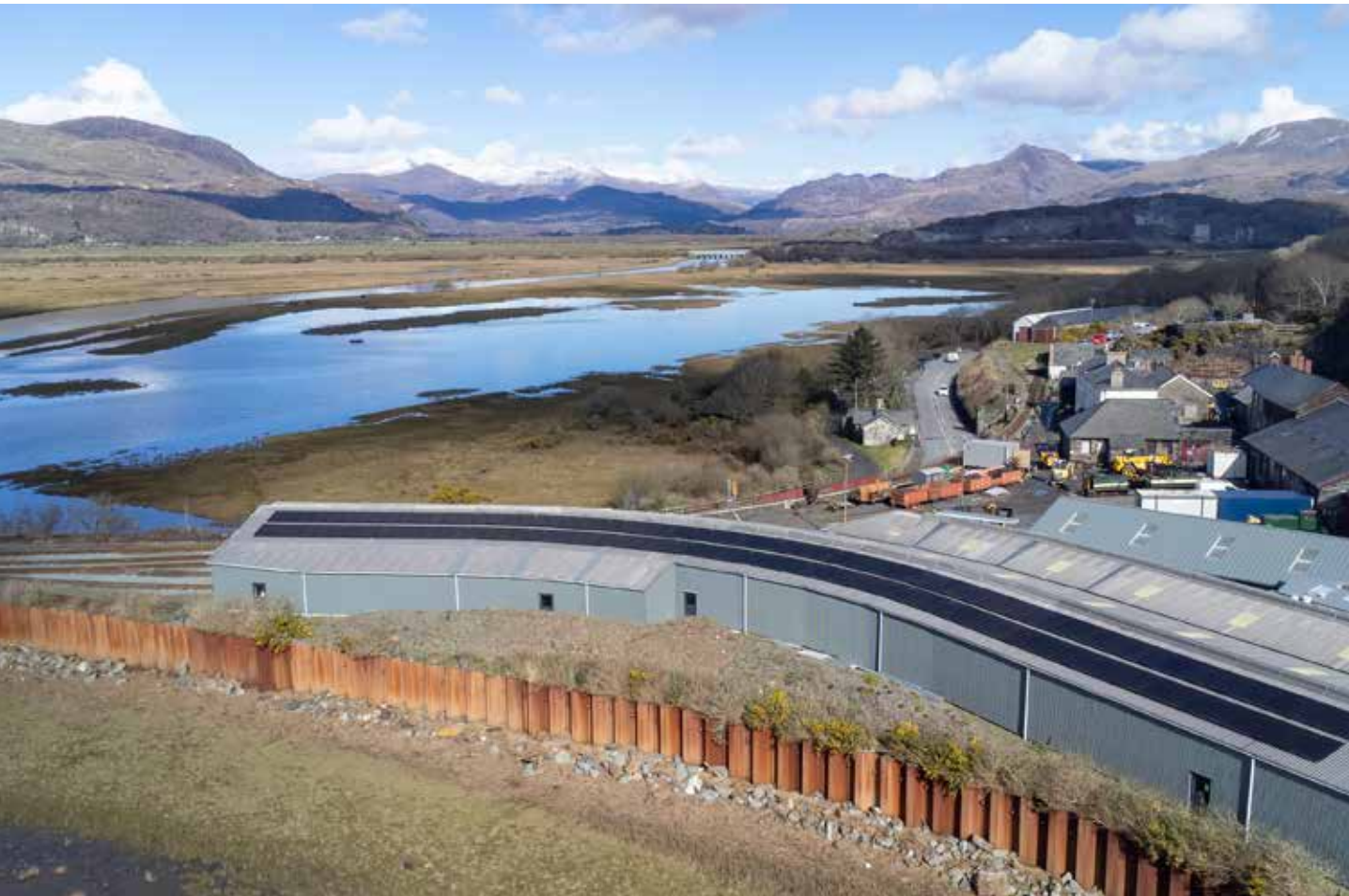
A picture from shortly after the install of the Solar Array at Boston Lodge Solar Array. Chris Parry
